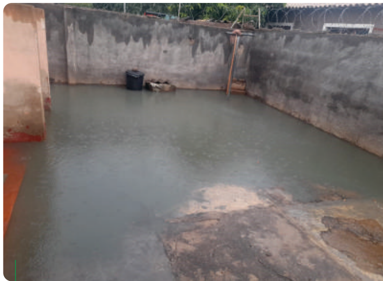
Picture of sewage overflowing into a house in Emganwini
